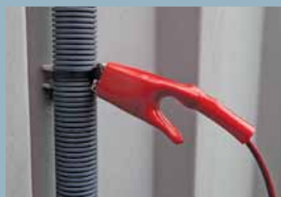
Small diameter cable tracing techniques
